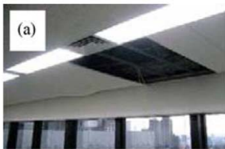
(a) Falling of ceiling at story levels 28, 21, 14, etc.
