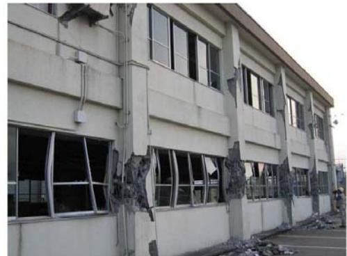
Shear Failure on Short Column (2004 Niigata-ken Chuetsu EG)
