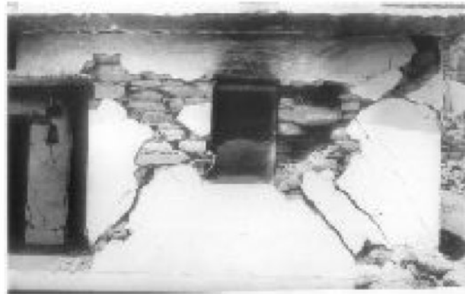
Figure 0.33 Extensive diagonal cracks in masonry walls (Ref: www nicee.org)
